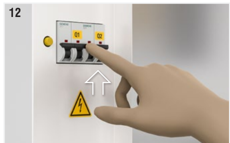
Fig. 12: Check that the magnetothermic switches for disconnection of the fan power supply (Q1) and for disconnection of the auxiliary power supply (Q2) are in the ON position.
