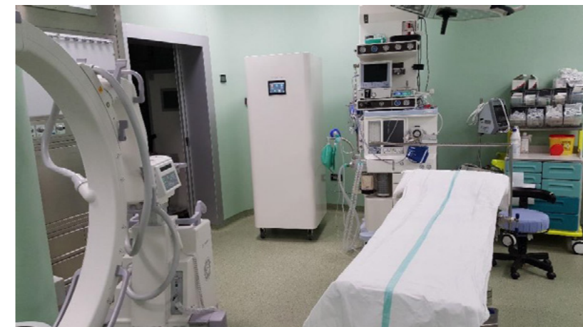
Photo 1 - Position of MATE cabinets inside the operating rooms
